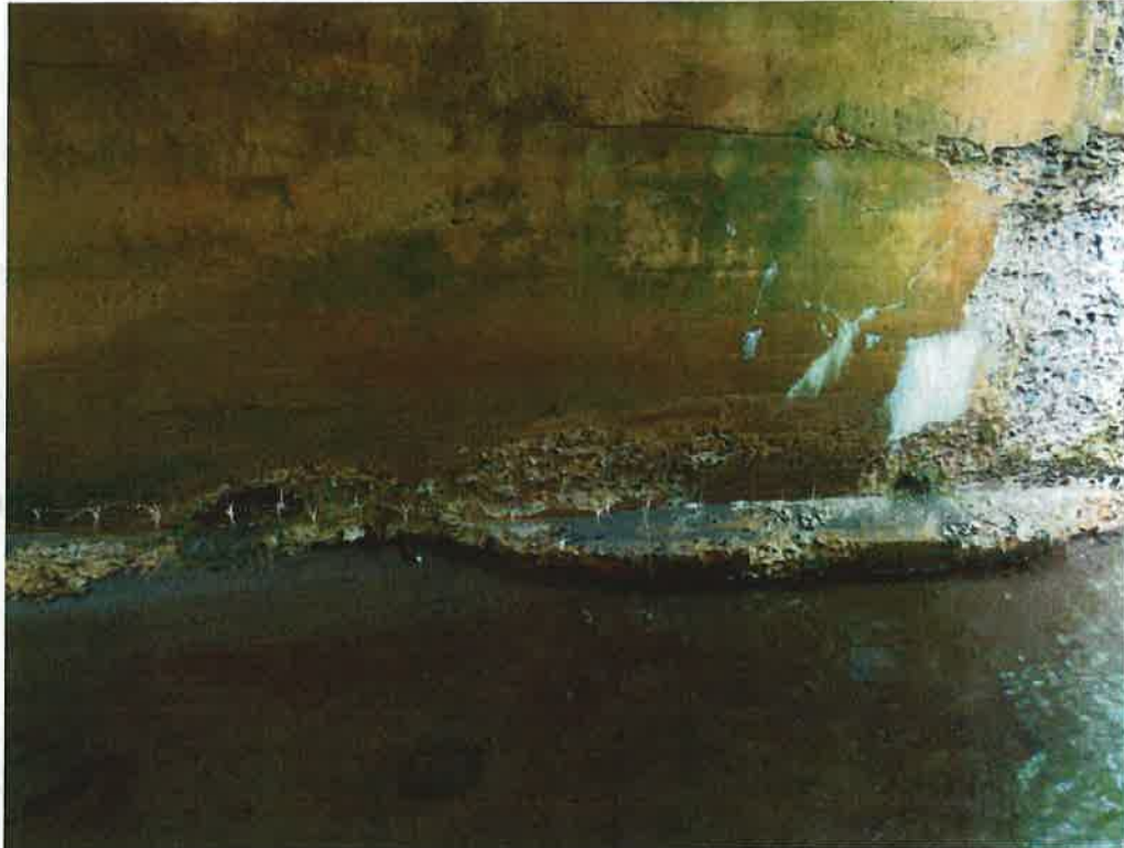
Photo 9: South breastwall with exposed footing and voids.
