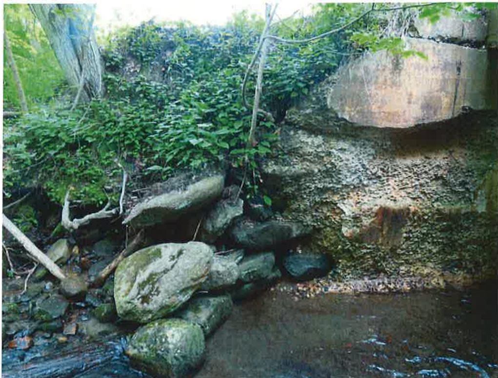
Photo 12: Northwest embankments with displaced stones & embankment erosion. Also note, wingwall/breastwall with severe scaling.
