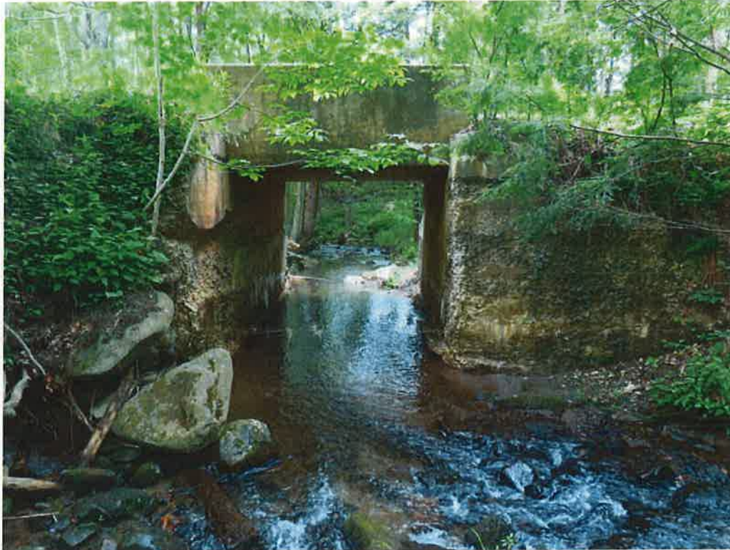
Photo 3: West elevation. Note, displaced stones and severe scaling of wingwalls.
