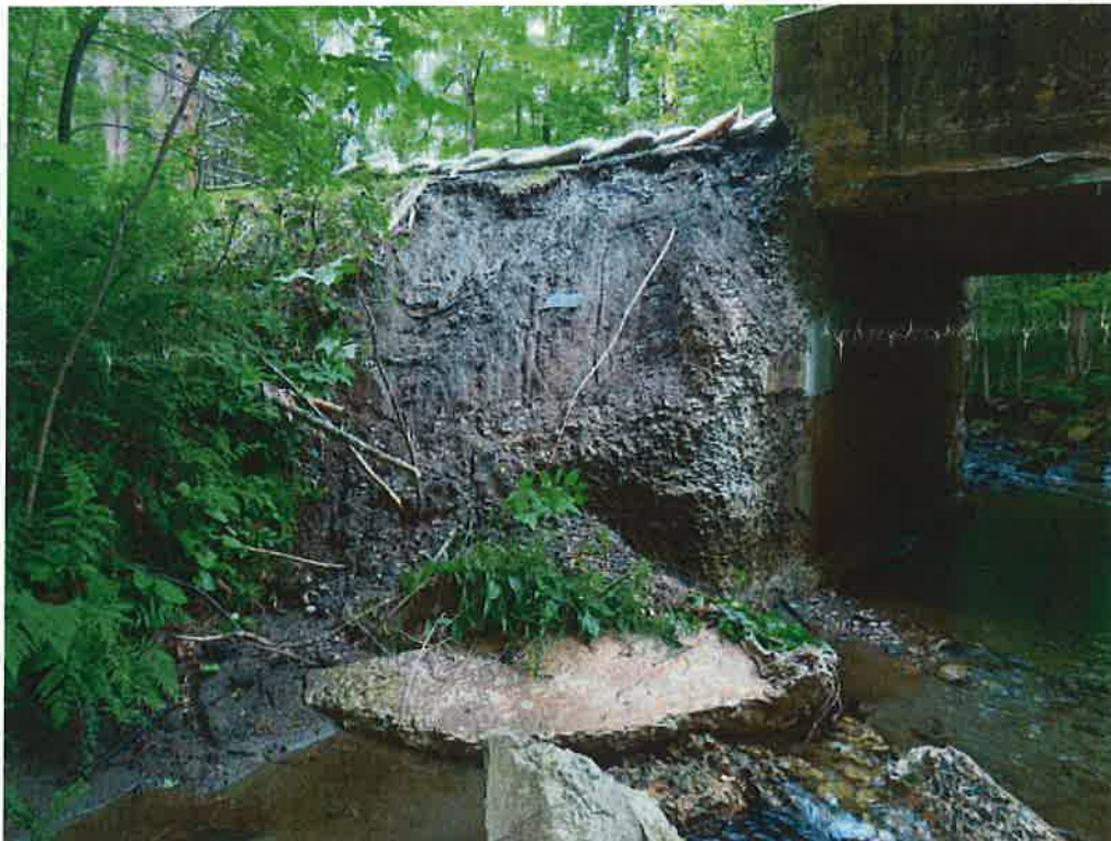
Photo 10: Close-up of southeast wingwall, failed.
