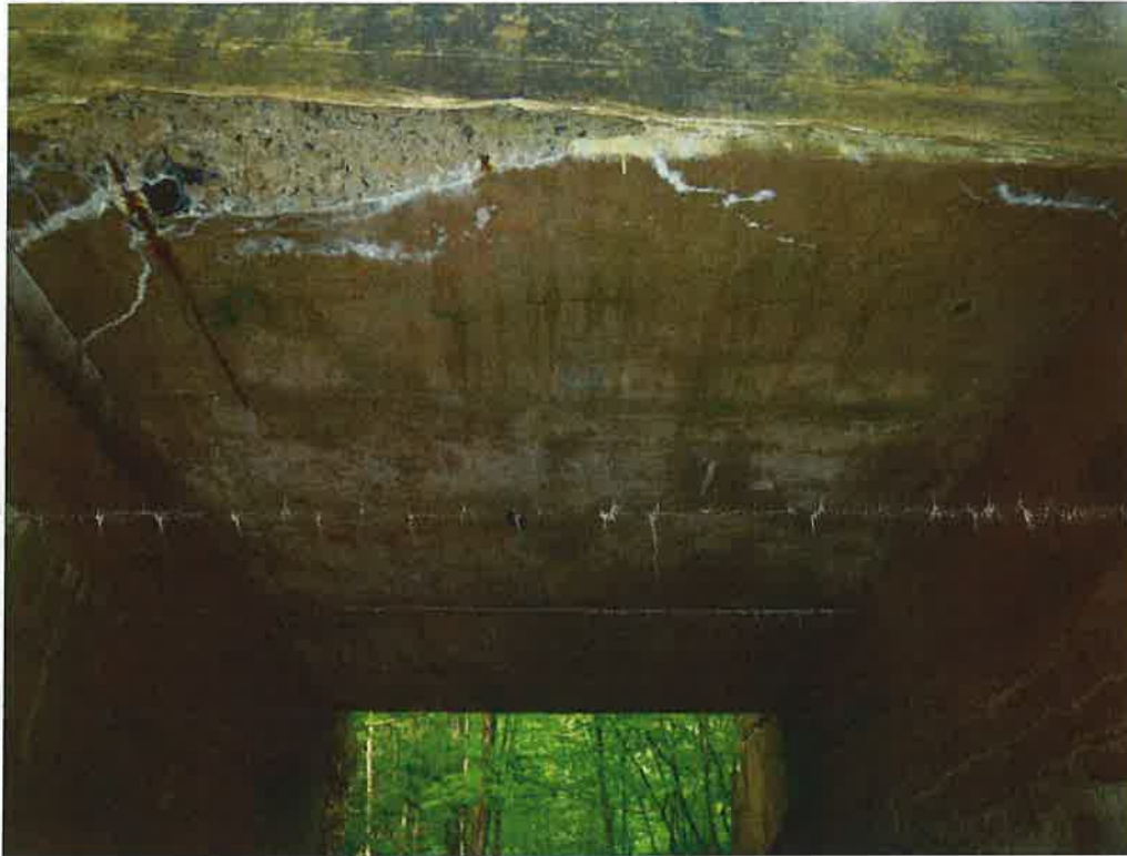
Photo 5: General underside view, looking west. Note, spalled area along the east edge.
