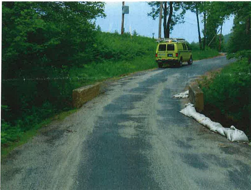
Photo 2: South approach. Note, sandbags at failed slopes.
