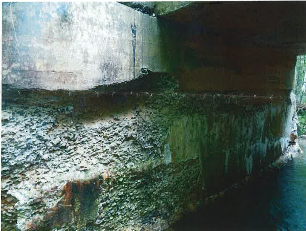
Photo 8: North breastwall with severe scaling, cracking and efflorescence.
