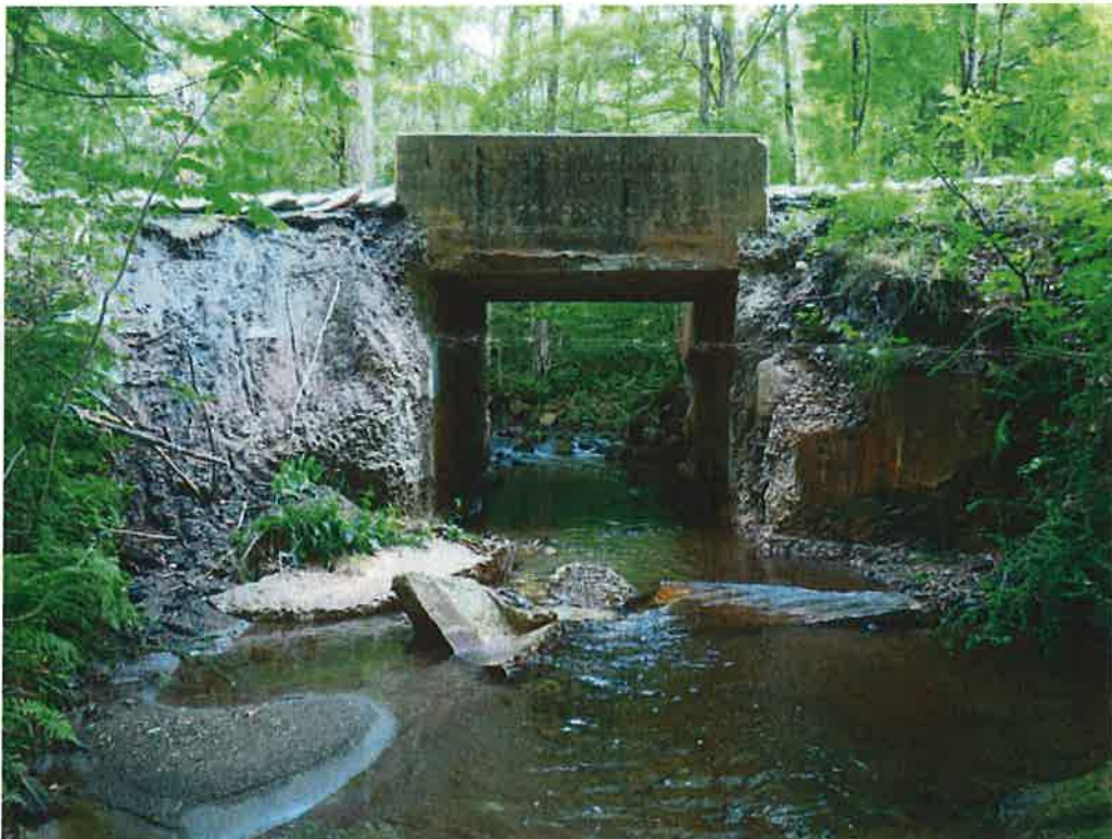
Photo 4: East elevation. Note, failed wingwalls in the channel.
