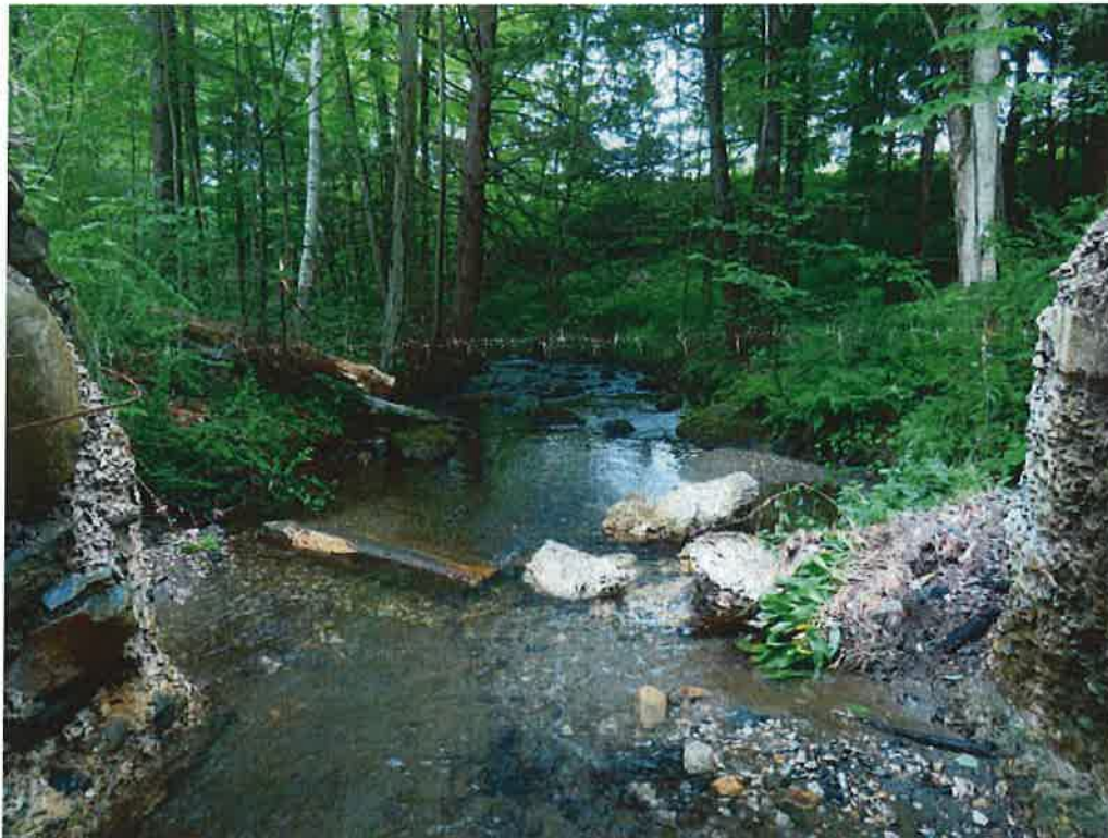
Photo 6: Downstream view. Note, failed wingwalls in the channel.
