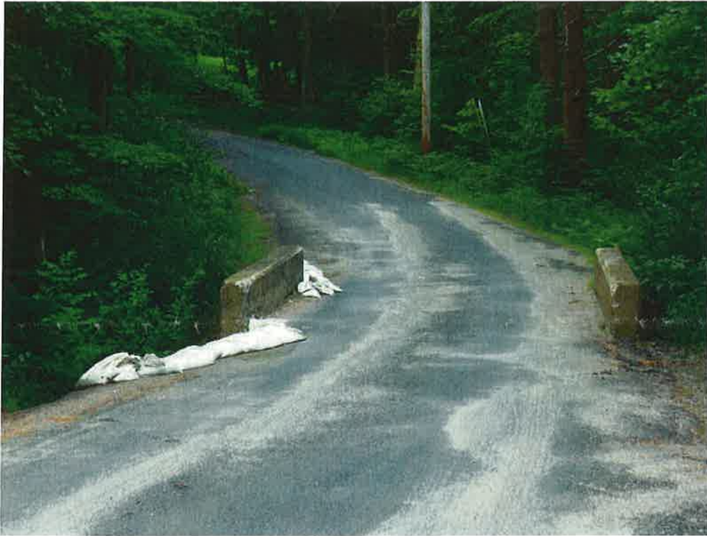
Photo 1: North approach. Note, sandbags at failed slopes.
