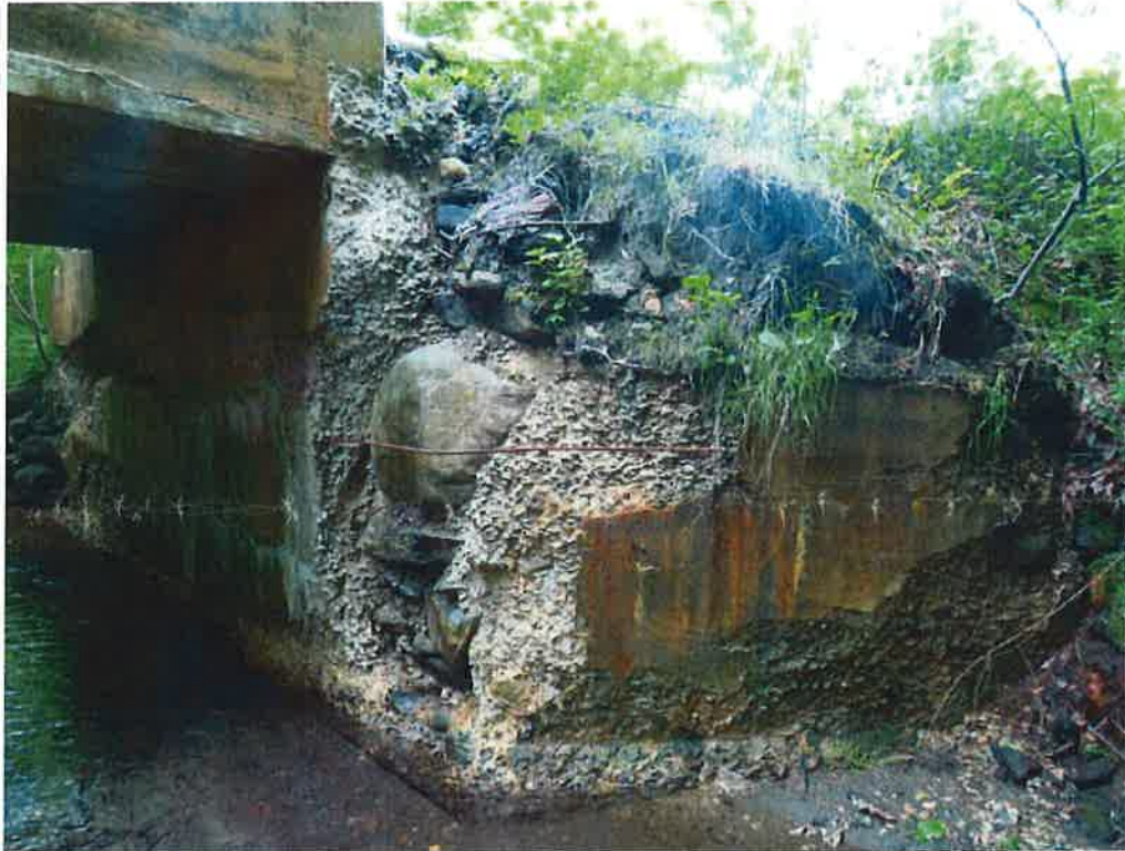
Photo 11: Close-up of northeast wingwall, partially failed. Also note, footing exposed and scaled.
